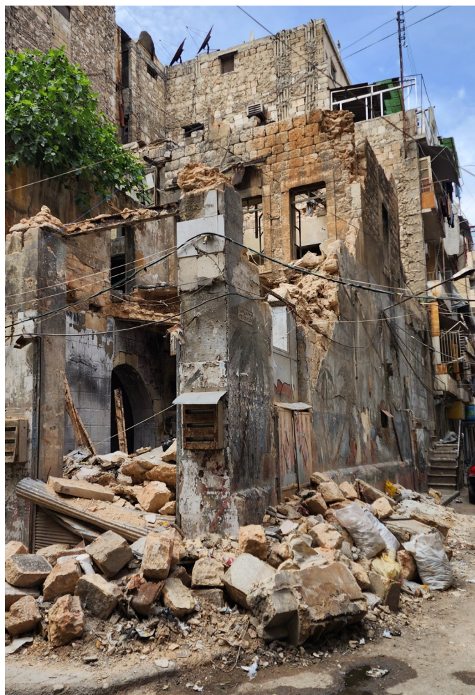
Devastation in Aleppo after the earthquakes
